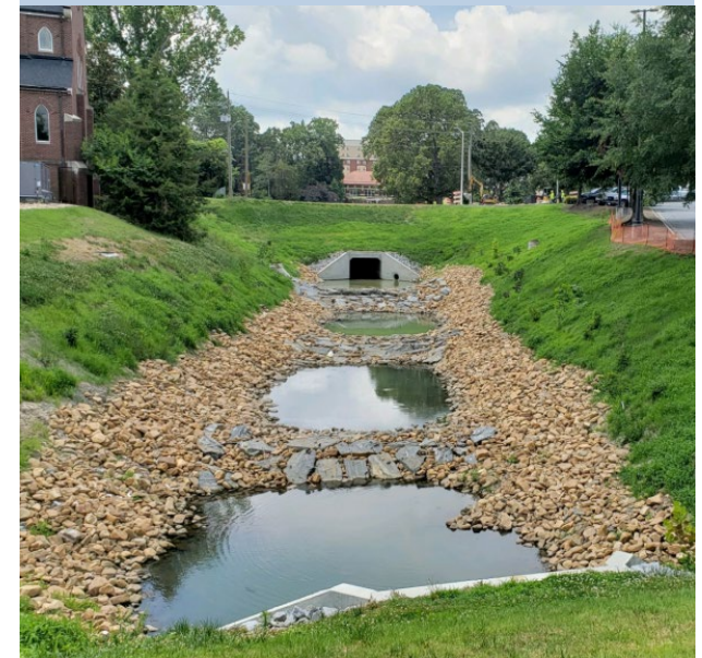
A regenerative stormwater conveyance system in Greenville, NC. Photo courtesy of WK Dickson & Co., Inc.
